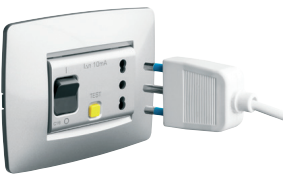
1- the absence of voltage on the holes is ensured.
