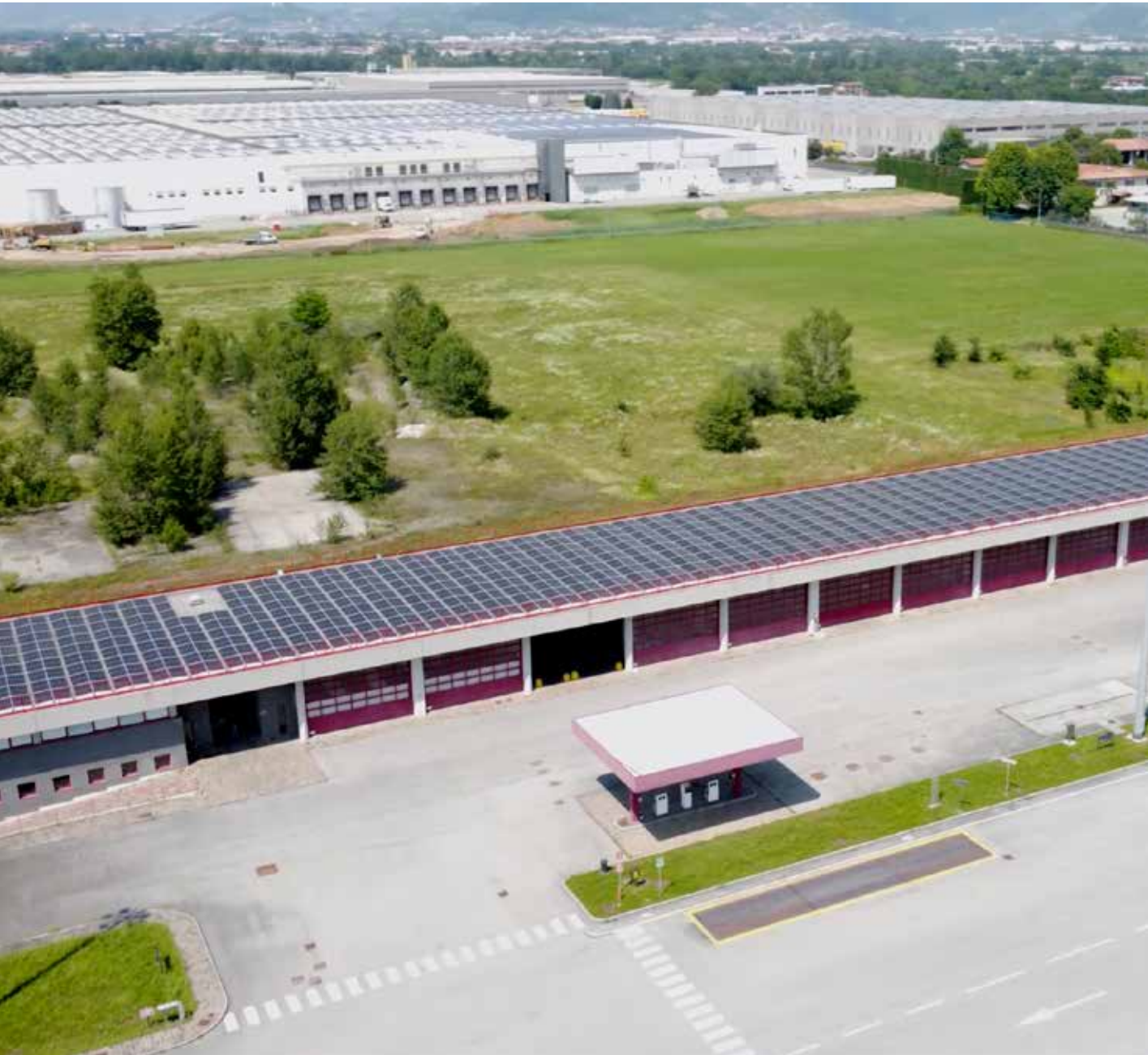
Calcinate photovoltaic plant (BG)
